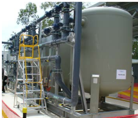
PRESSURE FILTER STATION
