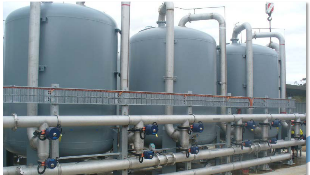
PRESSURE FILTER STATION
