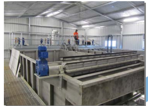
VIEW OF TOP OF DISSOLVED AIR FLOTATION FILTRATION TANK
