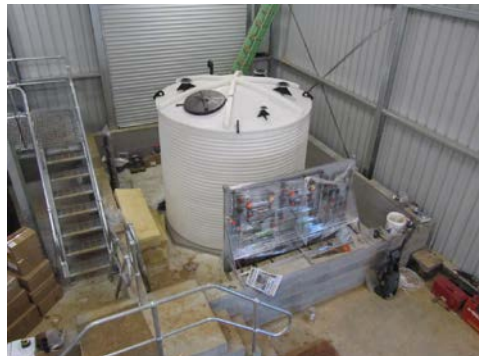
ALUM DOSING TANK & ASSOCIATED DOSING SYSTEM
