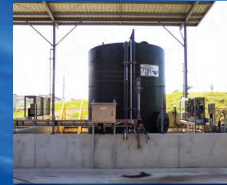
Ballina Wastewater Treatment Plant
