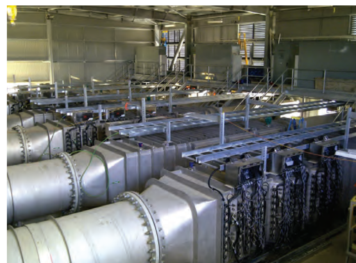
Eastern Treatment Plant WTP Torrent System
