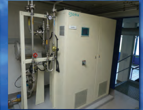
Rochester Water Treatment Plant
